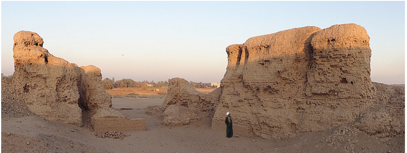
South face interior: The crack and south corridor at the start of the campaign.
