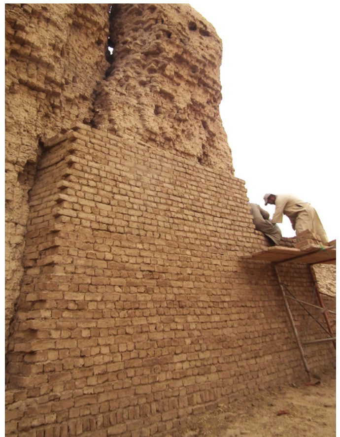
Bracing the breach: As high as we could get in a sandstorm.
