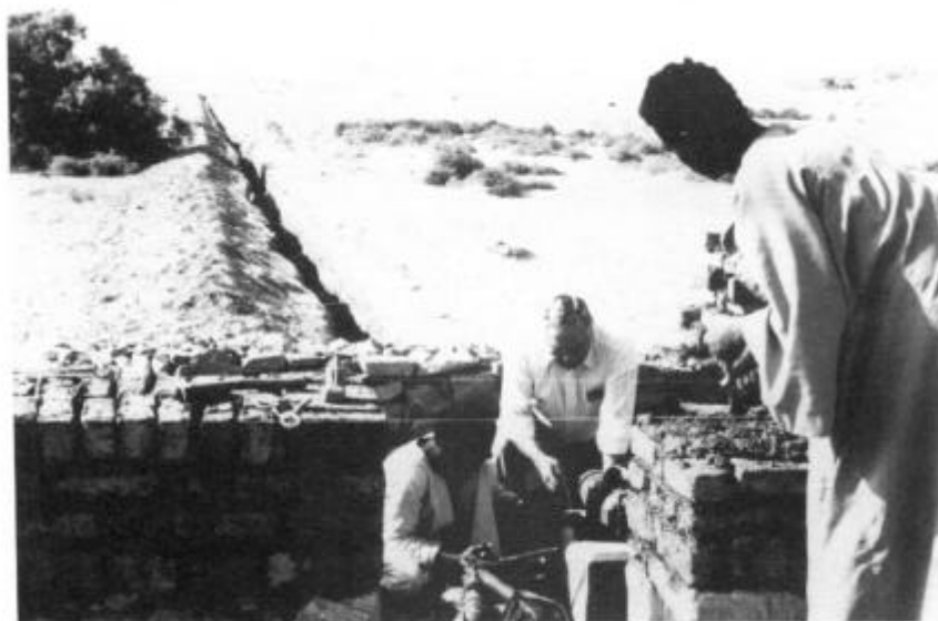
Tom Cox and crew at the water-pipe trench leading from the well to the walled compound.
